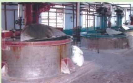
Critical down stream process facilities
